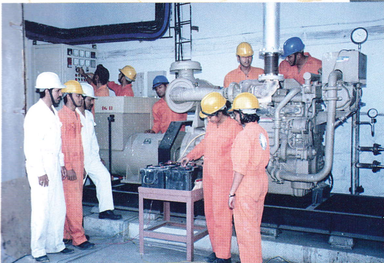
One of the two auxiliary generators - providing emergency power to the institute
