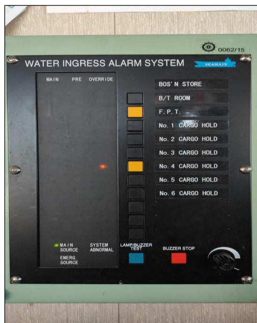
Fig. 2: WIDAS sensor alarm panel
