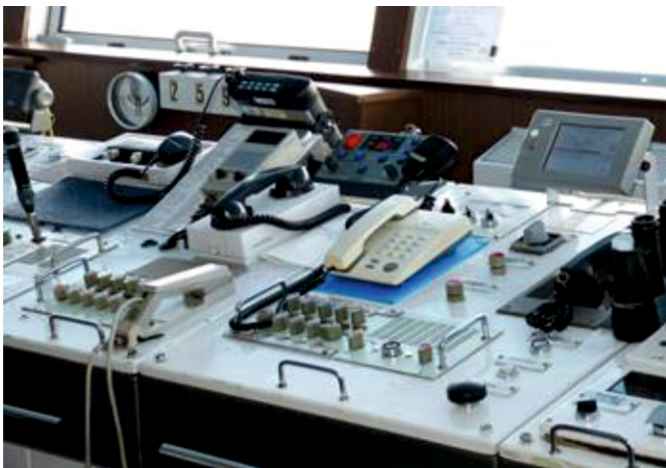
Fig. 1. Deck officers control room
