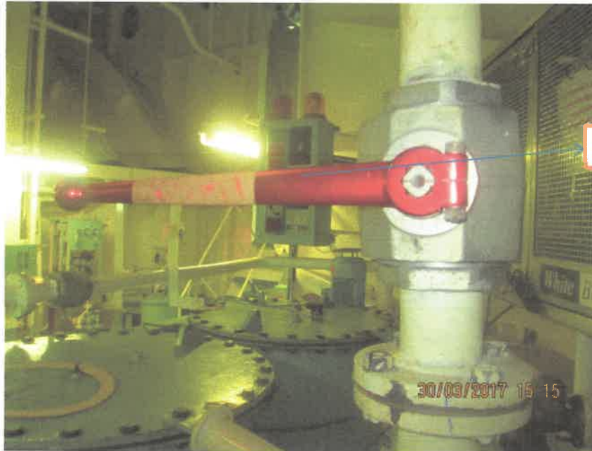
Outlet valve of white box
