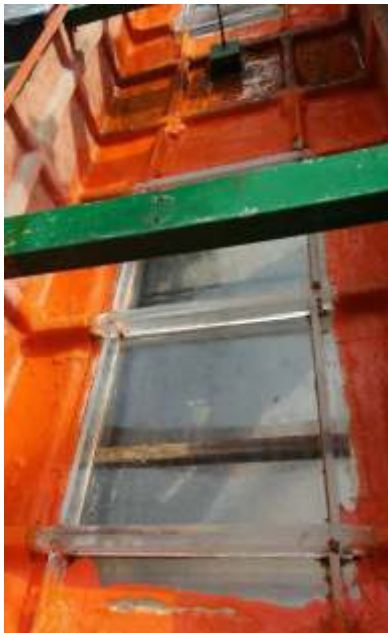
Fig. 9. Strengthening of acrylic frames with hull using GRP, putti and special adhesives
